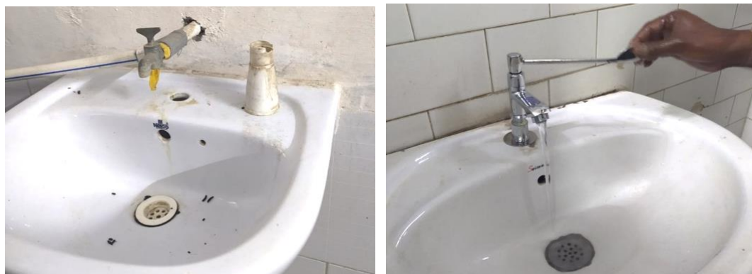
Before and after images. Installation of elbow tap (right) at Civil Hospital Ganjbasoda following dissemination of baseline results
