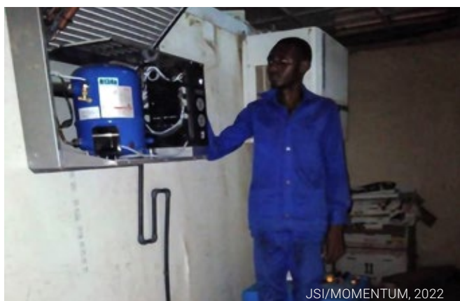
Project technician fixing a regional WICR.
