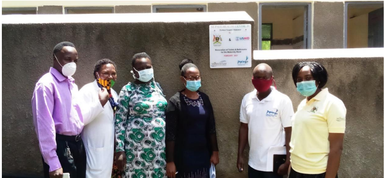
Lilian Biira (center) and MOMENTUM team members at the renovated toilet structure of the St. Paul's maternity ward. Photo: MOMENTUM Country and Global Leadership
