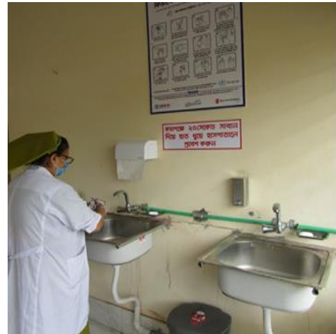
At sub-district level hospital, Staff nurse washing her hands at the Integrated Management of Childhood Illness (IMCI) corner which was installed by the MOMENTUM WASH/IPC project
