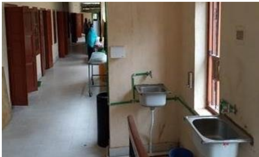
Newly installed handwashing stations at a facility in Bangladesh
